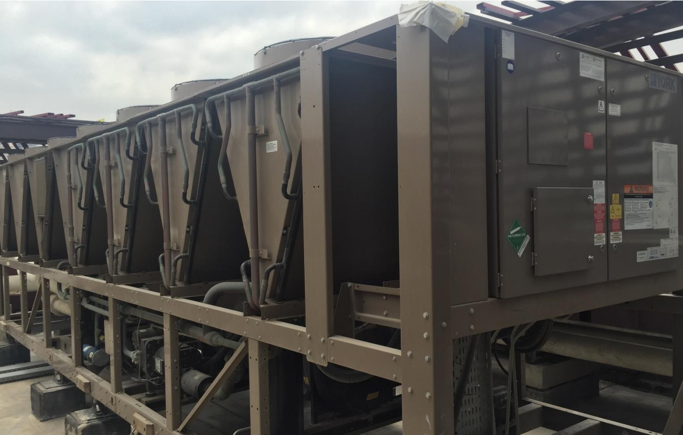
Efficient cooling system installed on the rooftop
