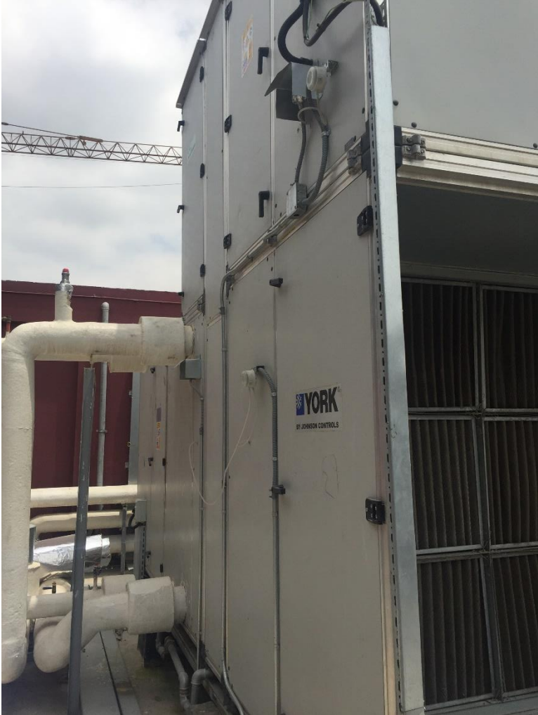
Efficient cooling system installed on the rooftop
