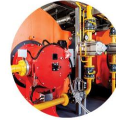
Steam Boilers 40.1 cross calorific value for lighth oil with 87% efficiency
